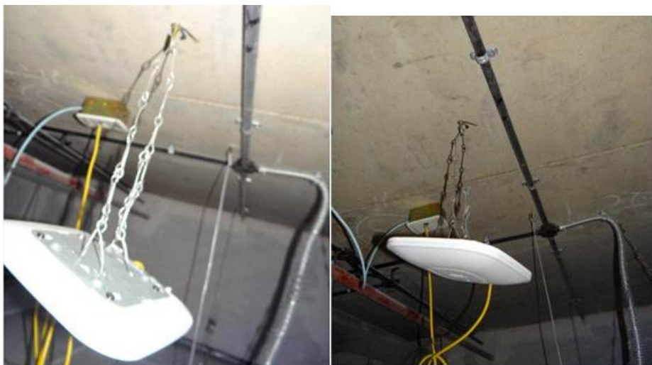
Figure 64: Improper Installation — AP not Level or Stable
